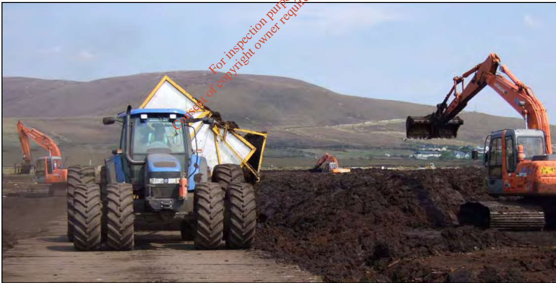
Plate 2: Peat unloading from Haku trailers onto deposition area (as part of the previous peat deposition operation on site, 2005 & 2007)
