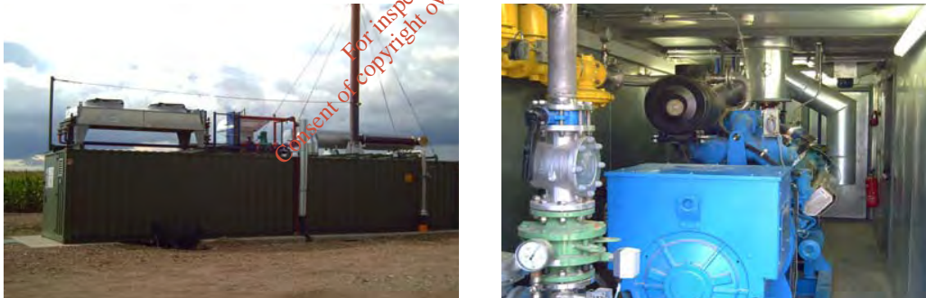
Fig.9. Containerised CHP at the Decker biogas plant in Northern Germany
