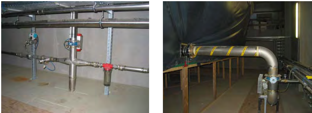
Fig. 8. The pneumatic gas collection system on the roof of the fermenters (left) and the gas transfer blower to the gas bag (right).
