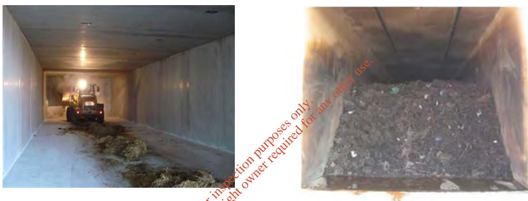
Fig. 4. Interior of fermenter prior to filling (left) and with bio-waste prior to fermenter sealing.
