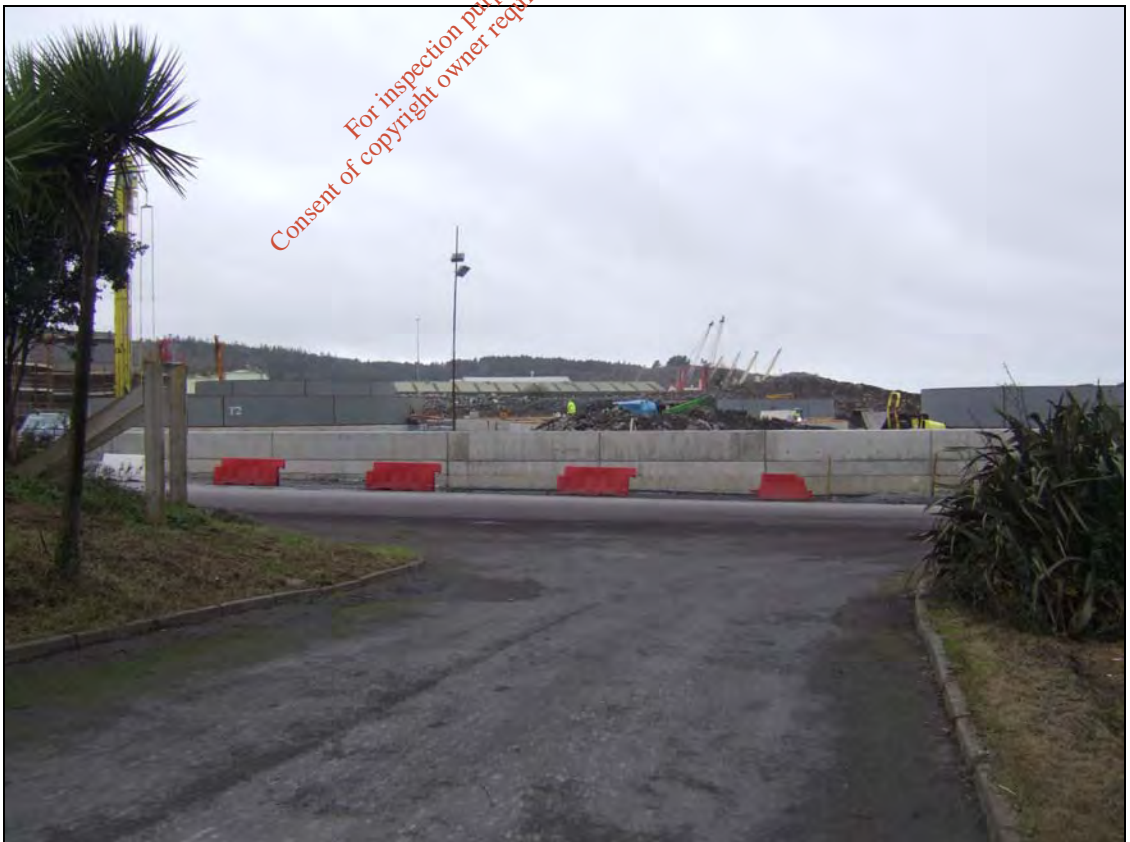
Plate 9.11 View of construction works within the Shannon Foynes Port Area from the site entrance
