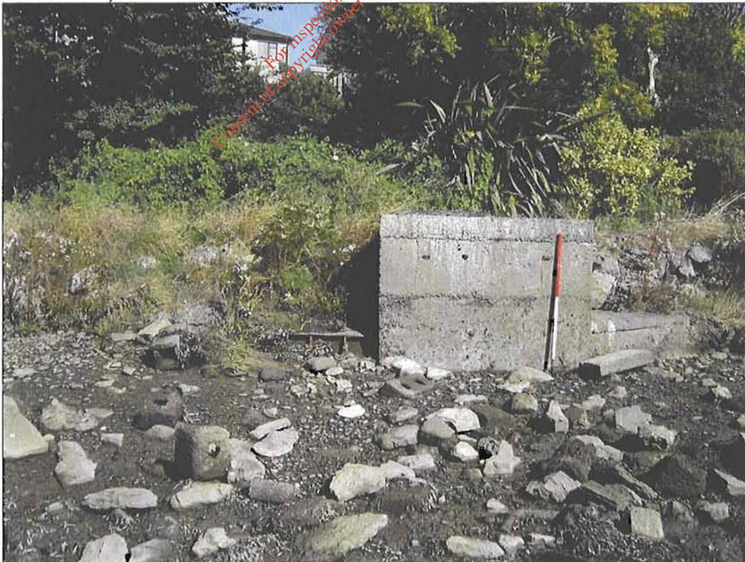
Plate 34: North-facing view of the upper foreshore c. 1860m along proposed pipeline route (see Figure 7 for location); 1m scale.
