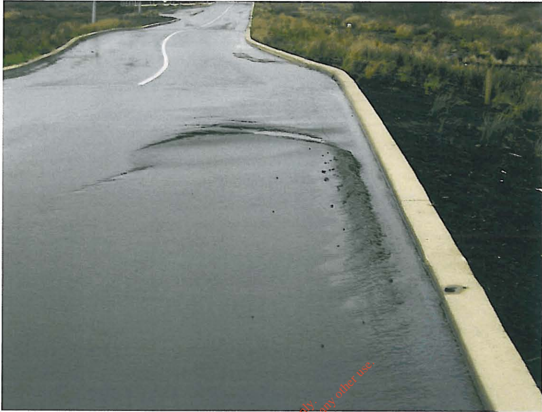
Localised cracks and rutting Haul Road
