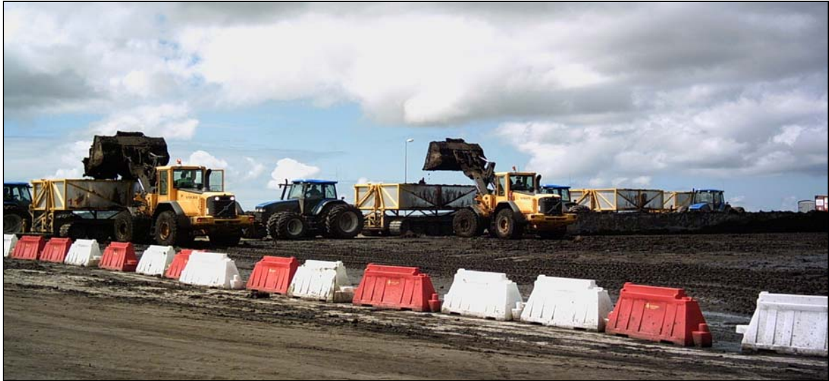
Plate 1: Loading of Haku Trailers from the Peat Reception Hardstand (as part of the previous peat deposition operation on site, 2005 & 2007)
