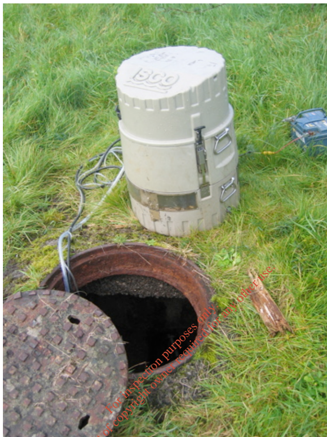
Plate 1: Rosses Point WWTP Influent Sampling & Flow Monitoring Location
