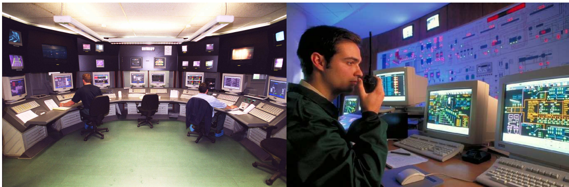
Figure 5.11 Typical Control Room and Control System
