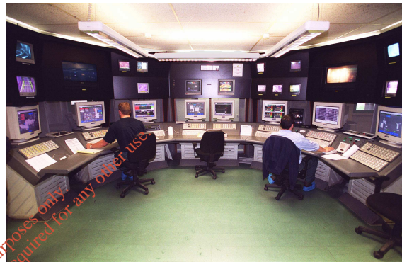
Figure 5.5 B) Control Room
