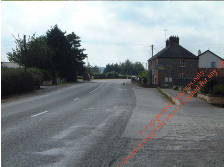
Photograph No 23 Carranstown Esso Garage Looking South (9.5m wide road excluding hard shoulder) (km 11.7)
