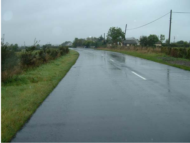
Photograph No 59 High quality section of R150 at Gaskinstown looking west, 2.5km west of Duleek
