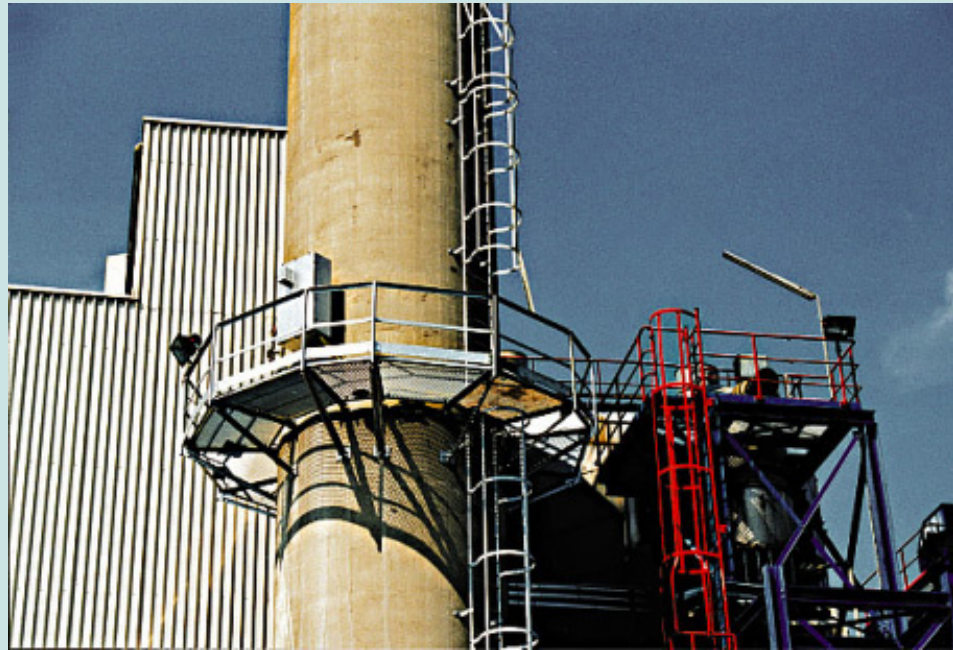
Outdoor-installation on the stack
