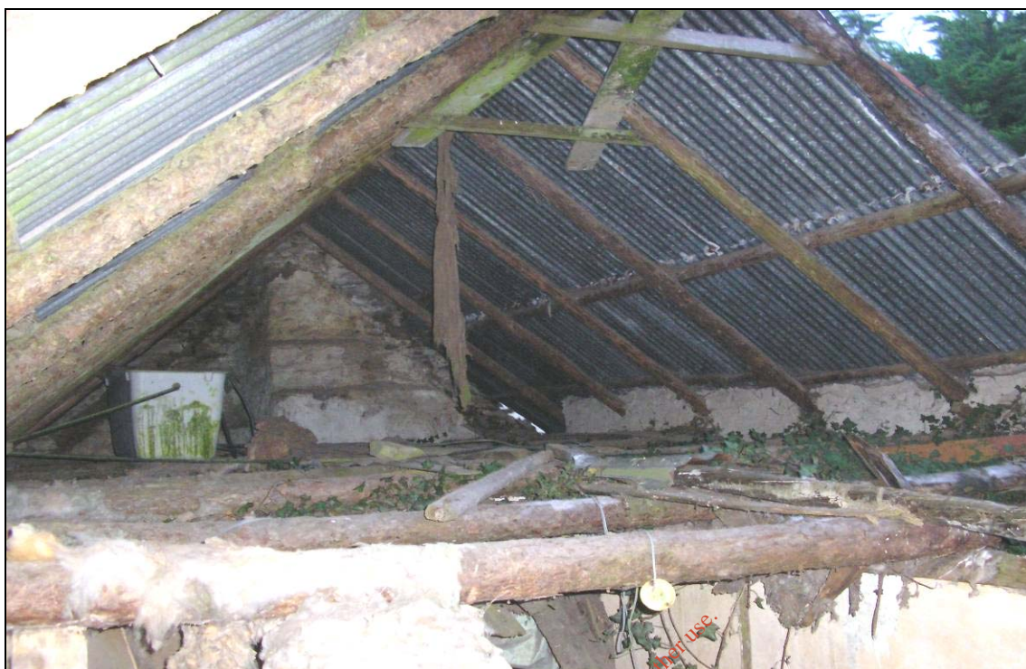
Plate 7. View within attic of derelict cottage.
