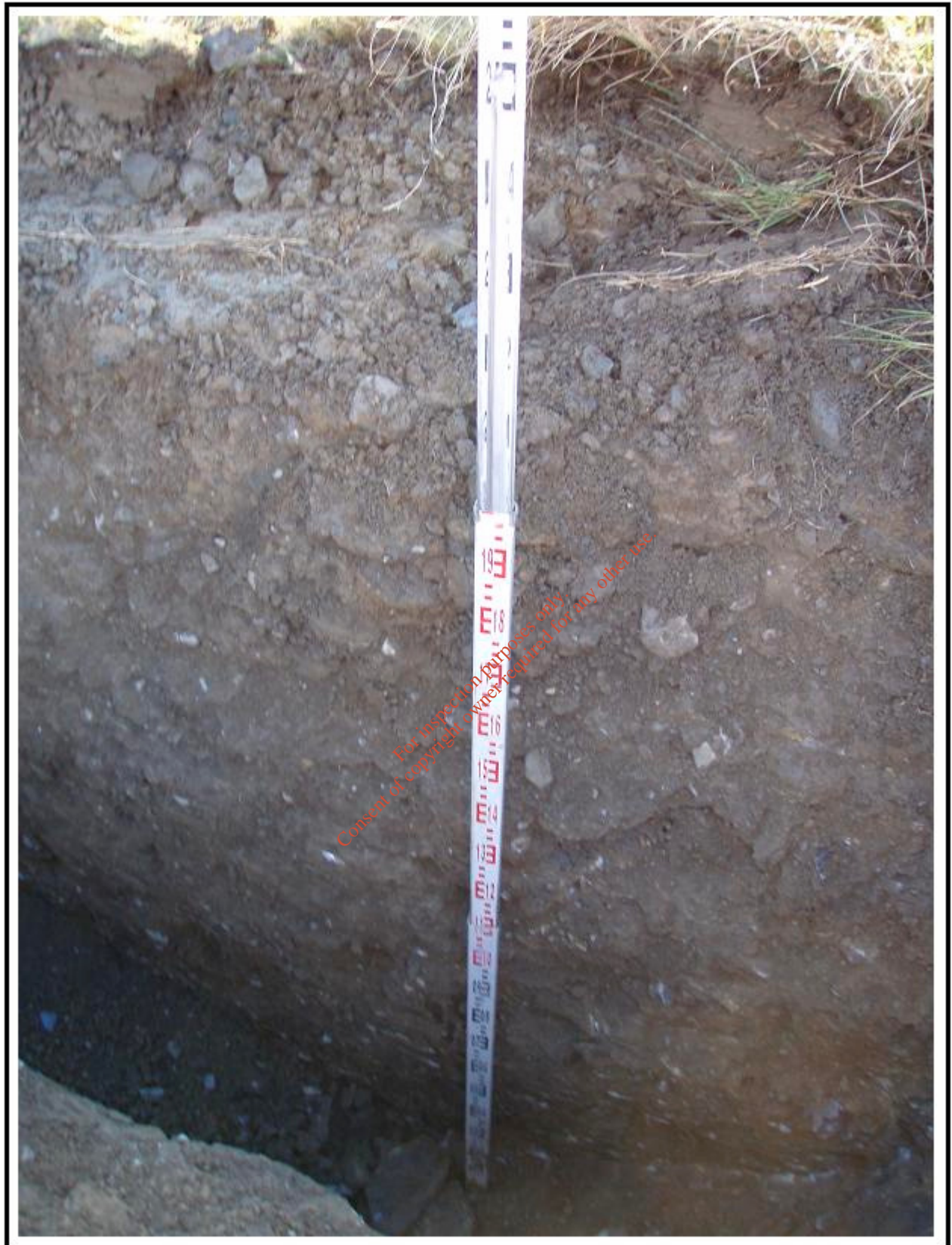
Plate A9: Profile of relatively shallow topsoil overlying overconsolidated, very stiff to hard subsoil in trial hole no. 9. See again the complete absence of waste material in the clean in situ subsoil here also. The topsoil is of very poor quality and may actually comprise mostly CLAY subsoil. The hole was dry to 2.2m depth.
