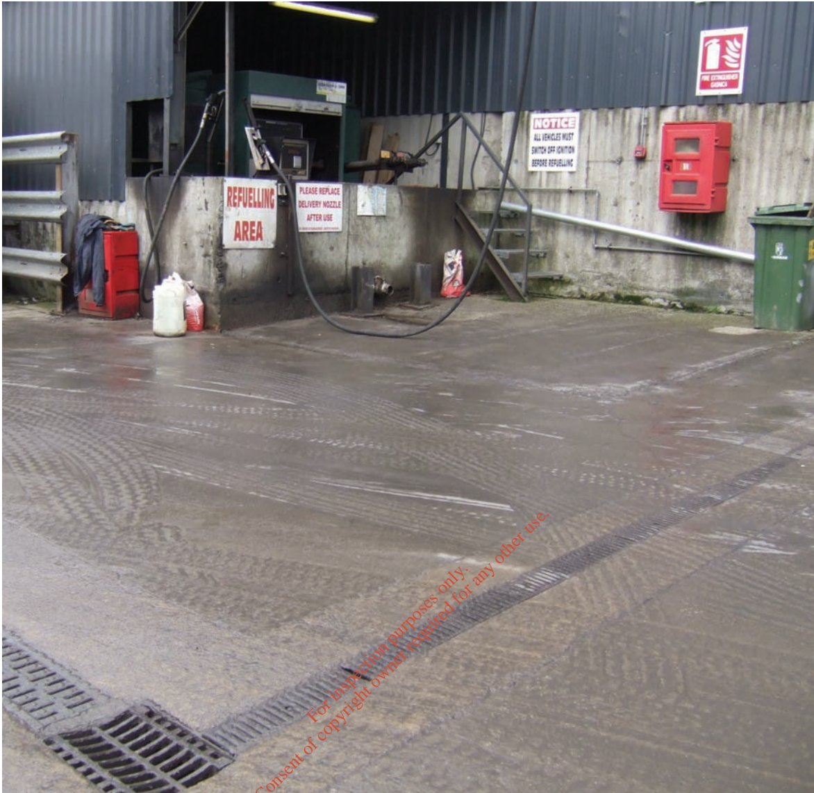
Plate 3.14 Onsite bunded fuel tank and refuelling area
