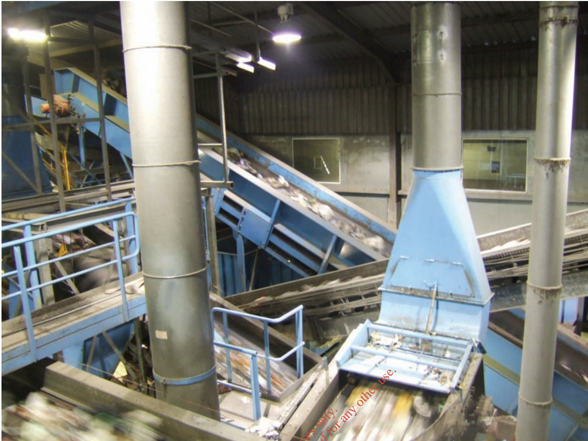
Plate 3.2 Conveyor belt system within MBT plant
