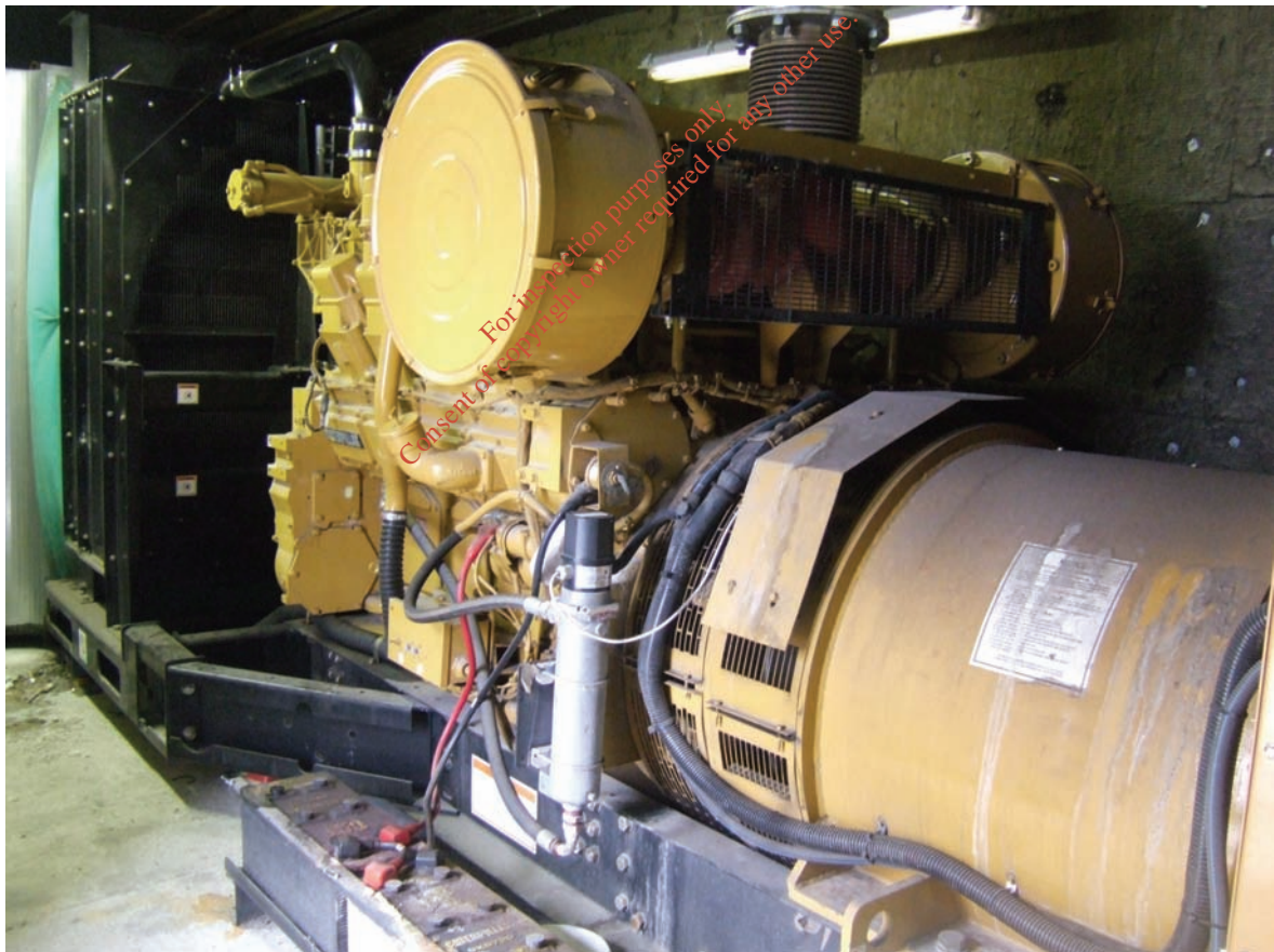
Plate 11.1 Onsite generator at waste transfer station
