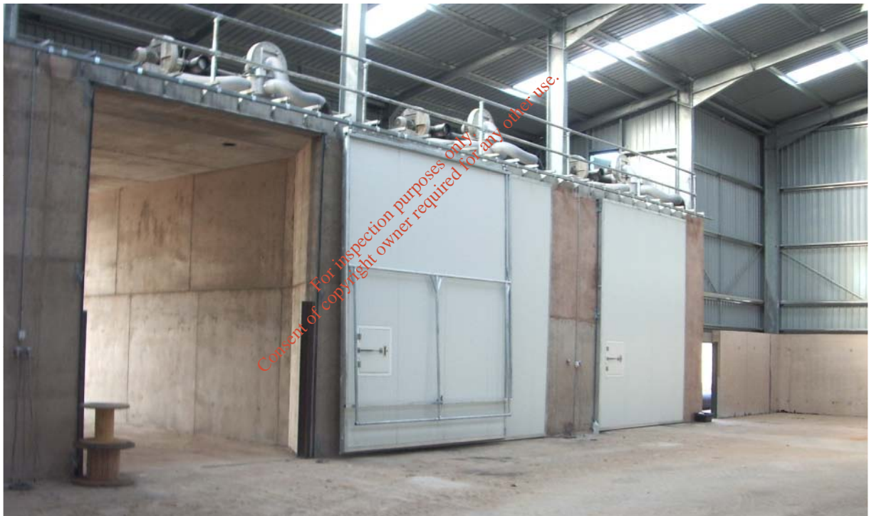
New concrete in-vessel composting system installed in County Devon, UK as seen from inside the tipping building
