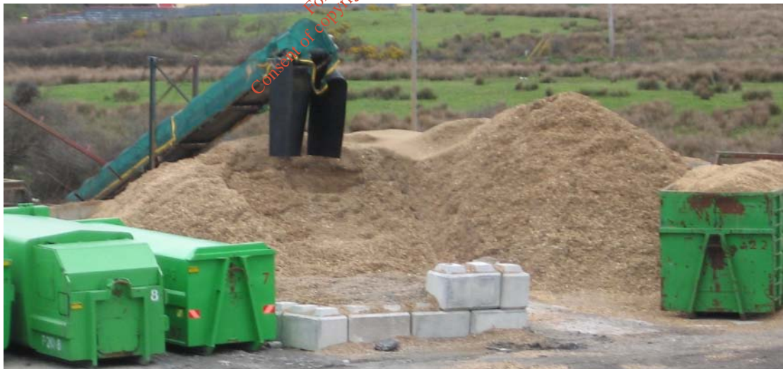
Top: Typical high speed shredder converting clean timber into wood chips. Above: Clean wood shredding area at CIRL site showing stockpile of processed wood chips. (Please note that a part of this overall planning and licensing application involves placing this whole shredding operation under roof.)
