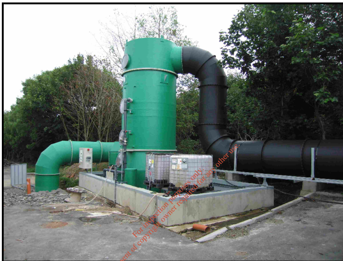
Plate 2.5 Typical scrubber configuration used to blend, humidify and scrub ammonia from the combined air streams.
