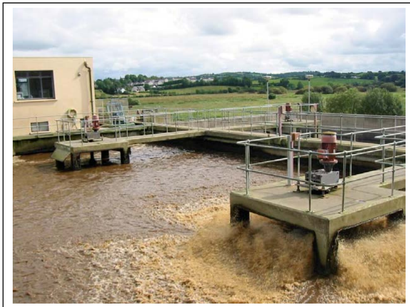
View of the Aeration System at Ballybay WWTW
