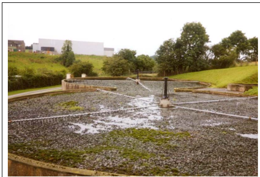
View of Bio-filter at Clones WWTP
