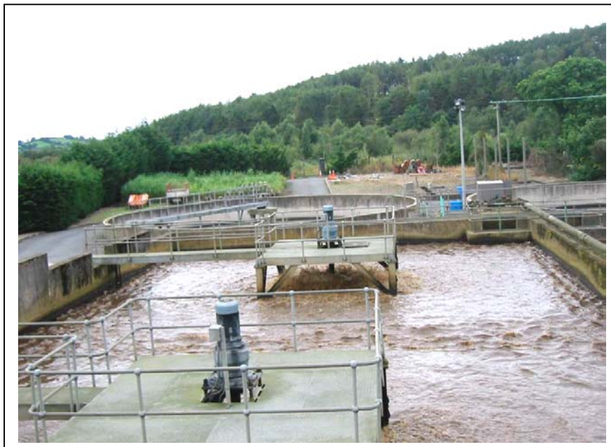
View of Aeration Tank at Castleblayney WWTP
