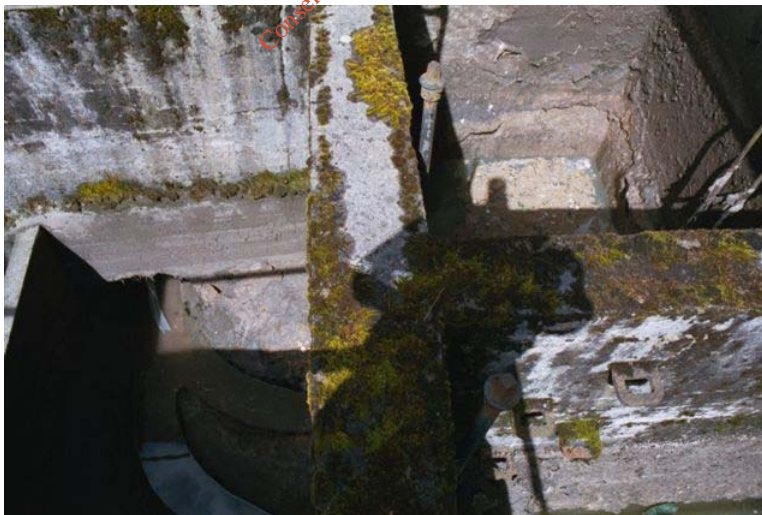
Figure SW03Dway-01 - Long Bridge Pumping Station
