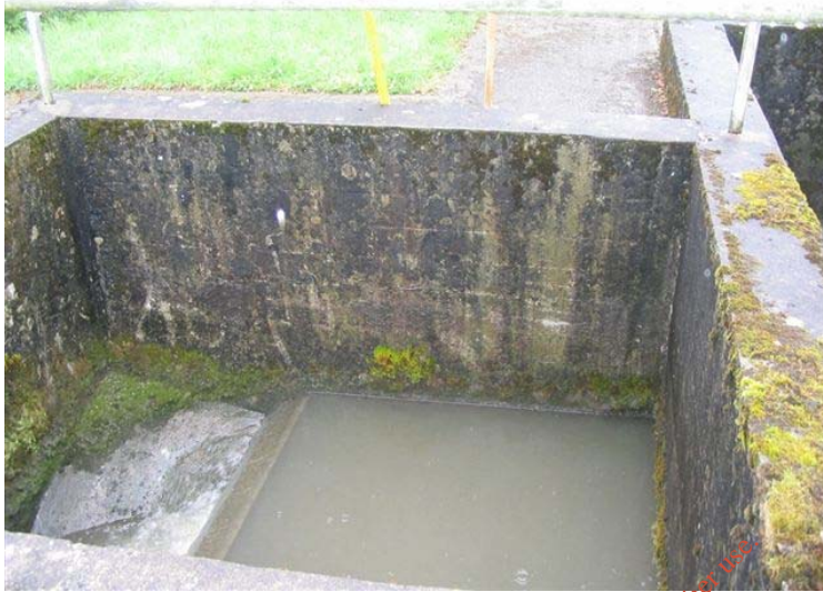
Figure SW05Dway-01 - Surcharged Inlet Quarry Road Pumping Station
