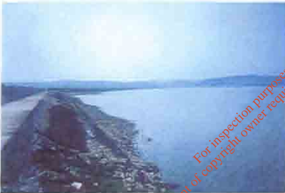
Plate B.3. The wall along the Youghal mudlands, showing the narrow biotopes along the wall.
