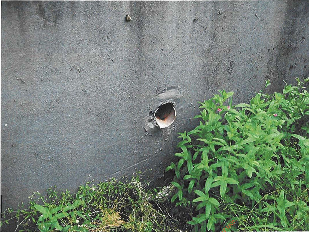
Emergency Overflow from Ballynamona Pumping Station
