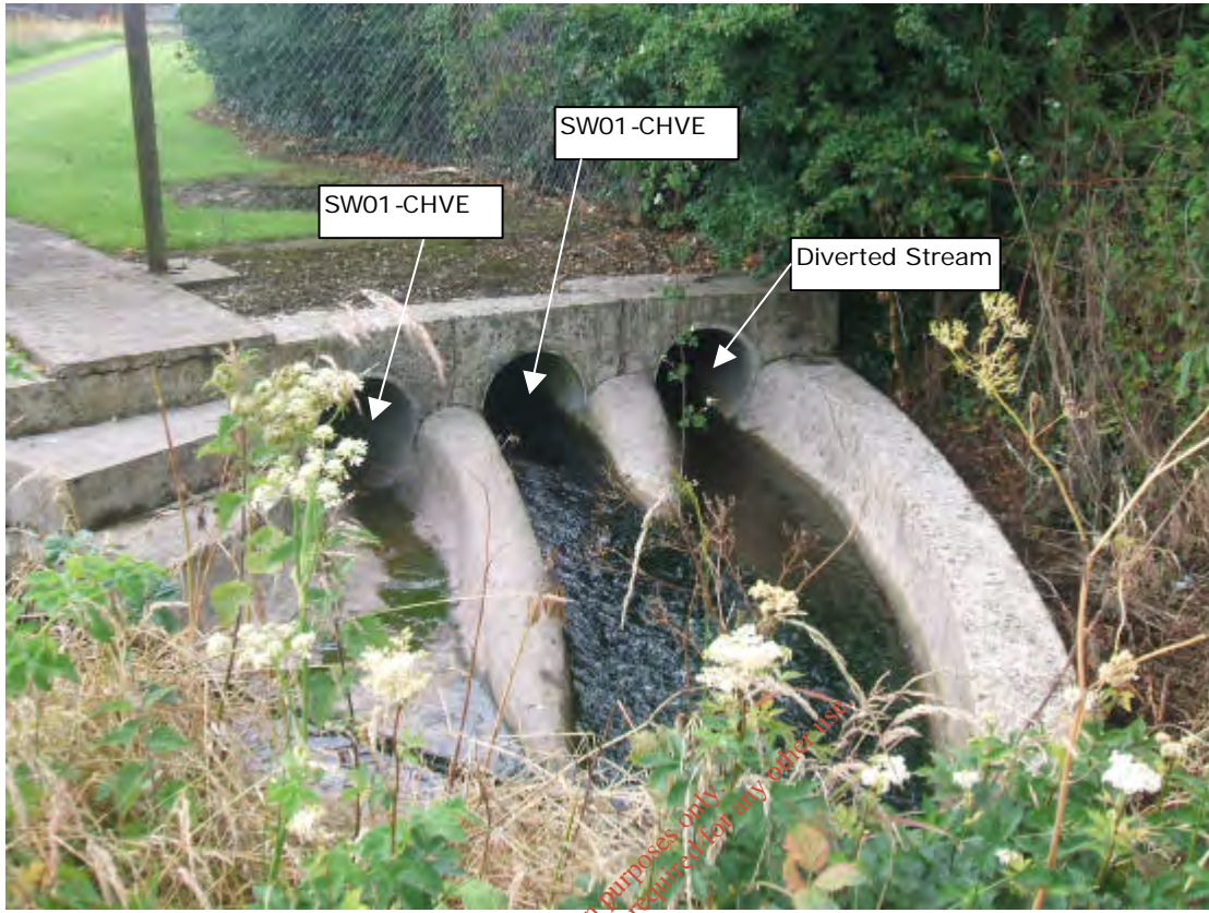
Photograph C2-01: SW01-CHVE, the primary discharge point from the treatment plant, and SW02-CHVE, the overflow discharge from the treatment plant
