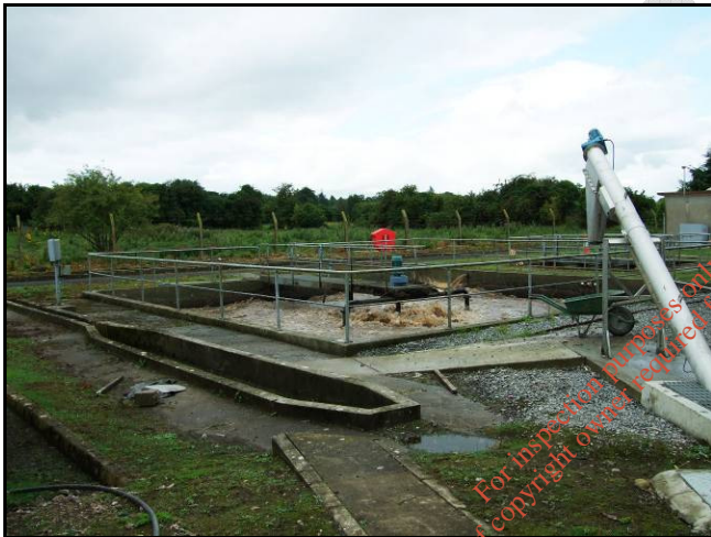
Plate 5 Activated sludge pond at the Abbeyleix WwTP.
