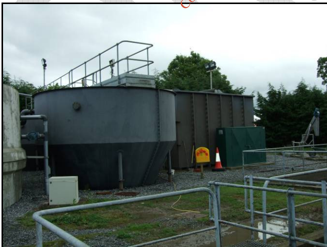
Plate 6 Rotating Biological Contactor (RBC) at the Abbeyleix WwTP.
