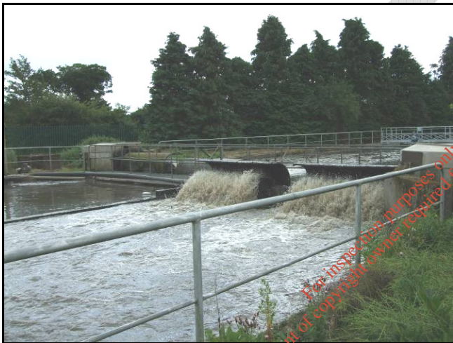
Plate 2 Activated sludge aeration at the Mountmellick WwTP.
