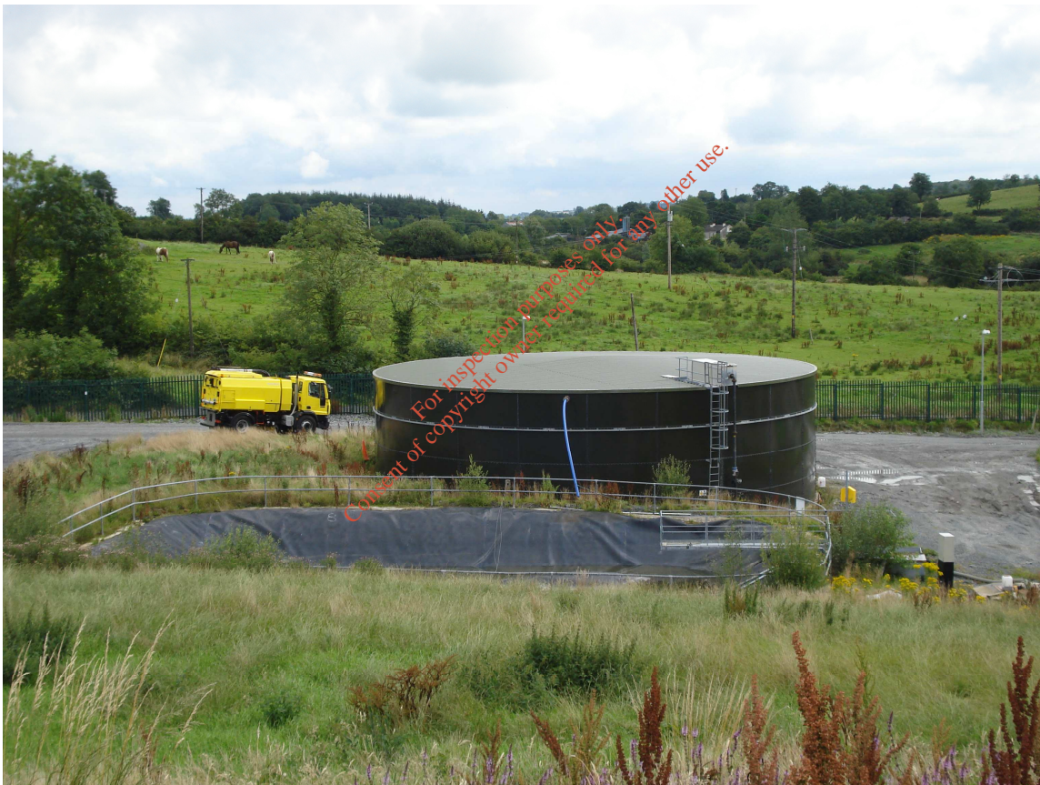
Figure 6 Leachate Storage Tank and Overflow Lagoon
