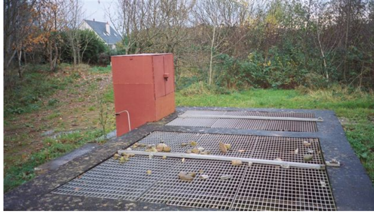
Photograph 3.7 Main IDA Pumping Station
