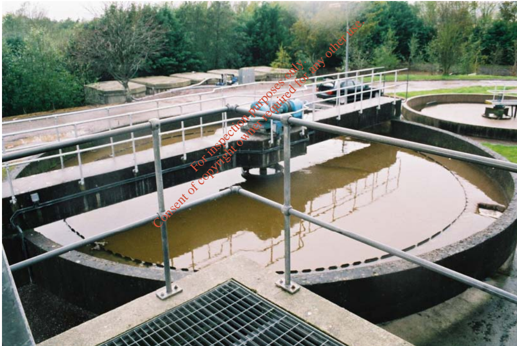
Photograph 3.5 Sludge Thickening Tank
