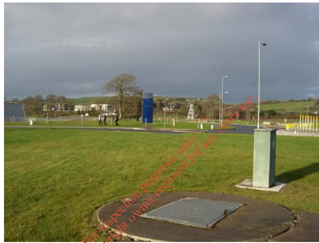
Photograph 3.8 IDA Pumping Station to North of railway Line
