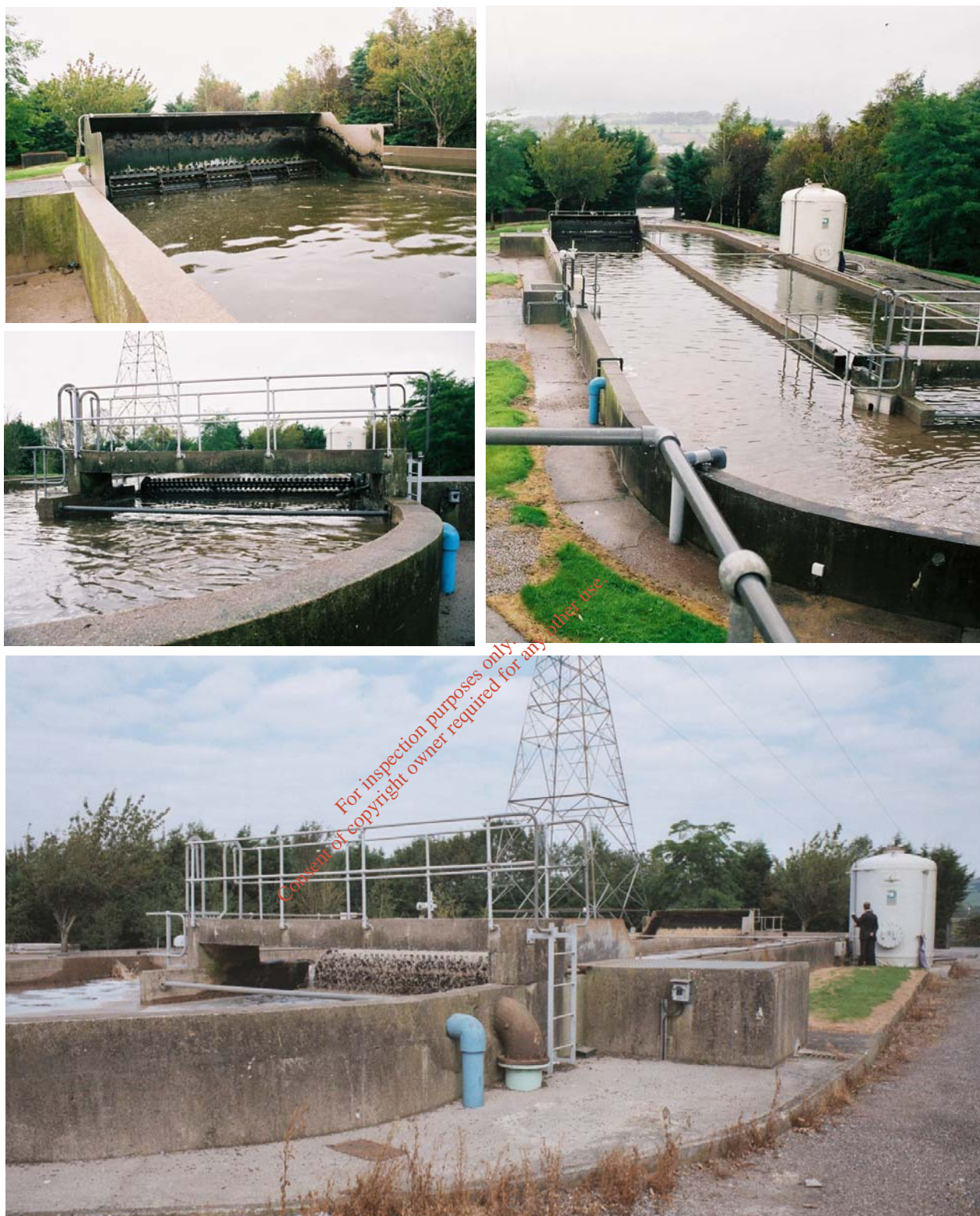
Photograph 1.3 Oxidation Ditch at Carrigtohill Works
