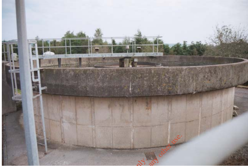
Photograph 3.3 Primary settling Tank at Carrigtohill works
