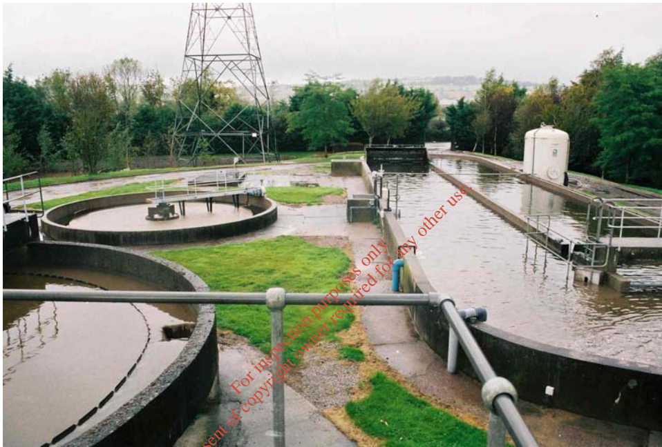
Photograph 3.1: View at Oxidation Ditch and Secondary Clarifier
