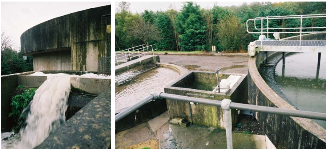
Photograph 3.2: Acid Dosing Chamber between PST and Oxidation Ditch
