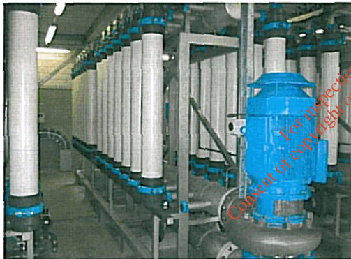
Figure 7: Overview of the nanofiltration plant ESSENT and a capillary module.
