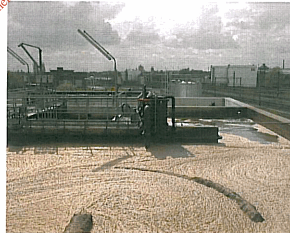
Denitrification (R), Nitrification (L) and carousel (in front)
