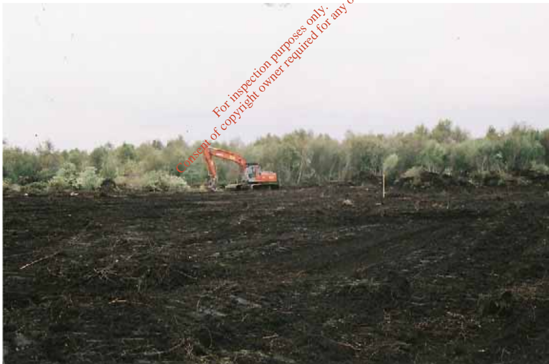
Plate 2. Stripping the cell of vegetation, note vegetation growth in background as an indication of how long the bog has been out of production.
