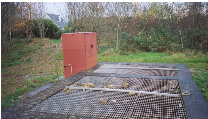
Photograph 3.7 Main IDA Pumping Station
