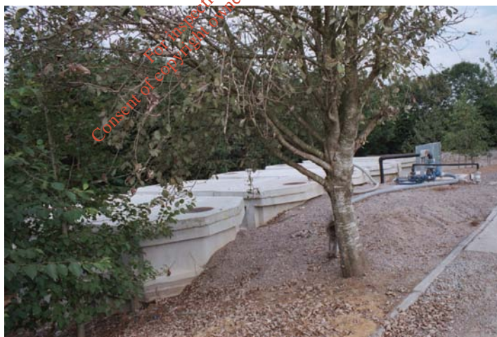
Photograph 3.6 Storage Tanks for Leachate from Landfill
