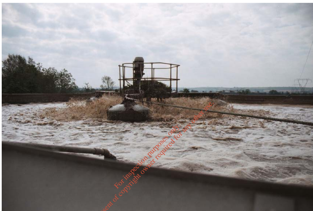
Photograph 1.2 Floating Surface aerator in Balancing Tank
