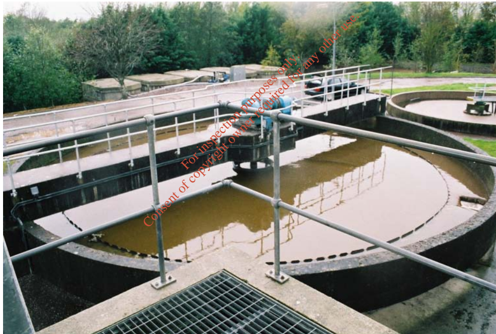
Photograph 3.5 Sludge Thickening Tank
