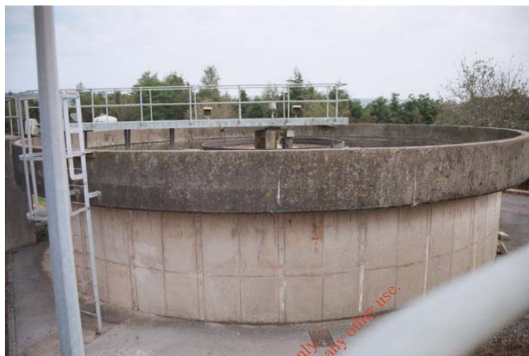
Photograph 3.3 Primary settling Tank at Carrigtohill works
