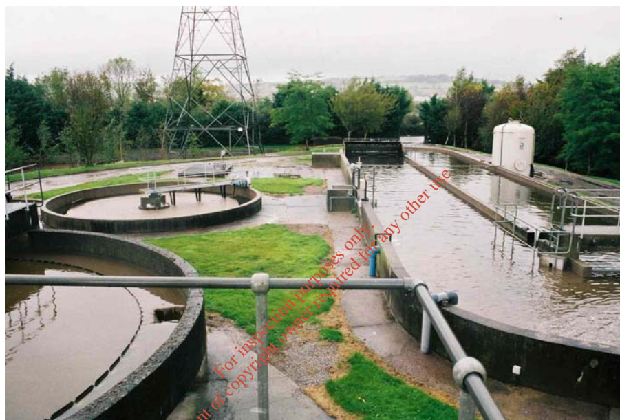
Photograph 3.1: View at Oxidation Ditch and Secondary Clarifier
