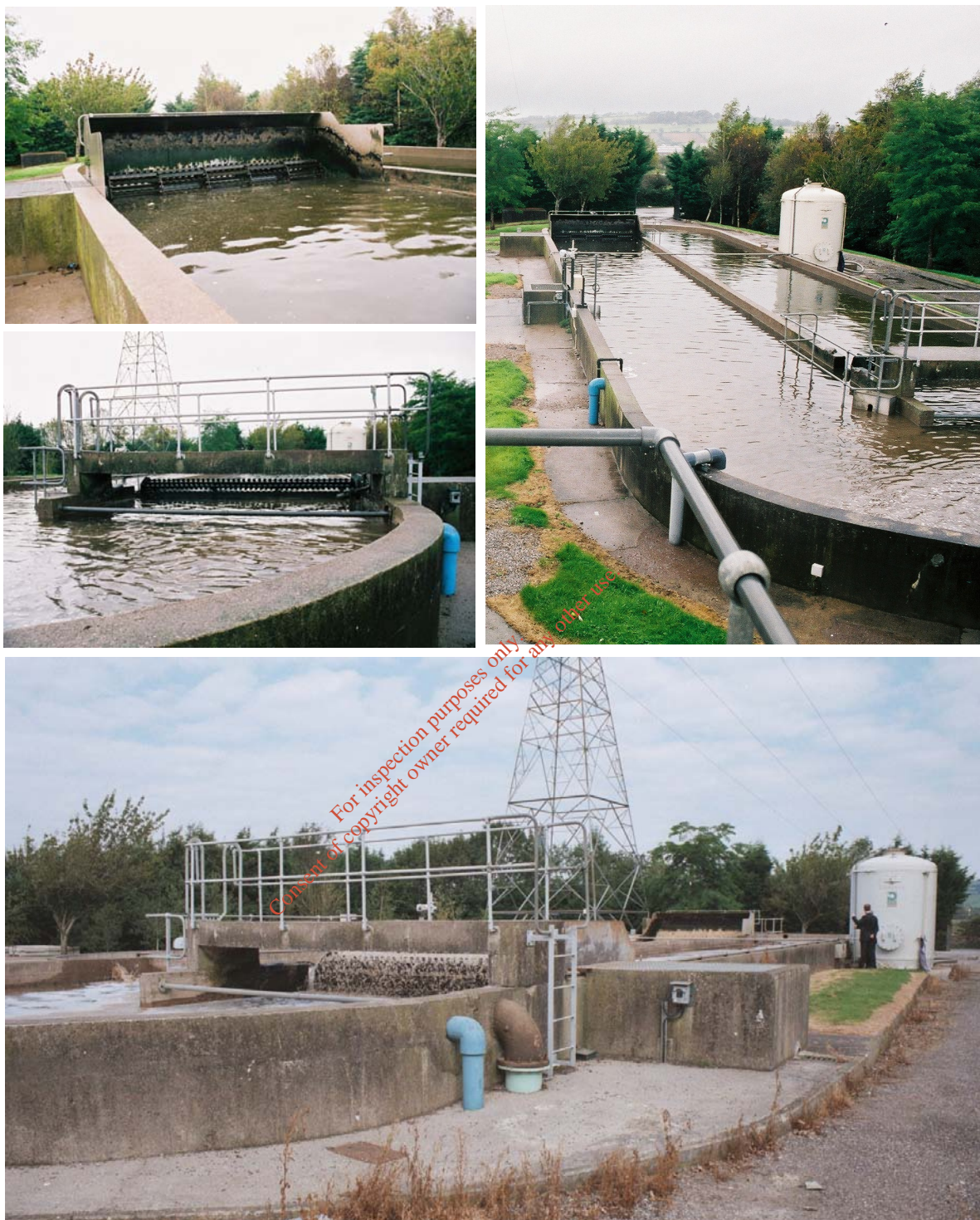
Photograph 1.3 Oxidation Ditch at Carrigtohill Works
