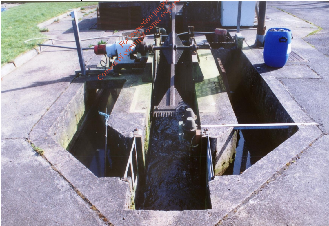
Figure 2.5 Inlet works with raked screen
