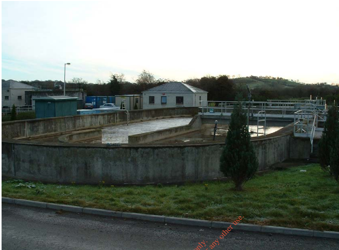
Photograph 1.1 – Aeration tank at the Carrickmacross works
