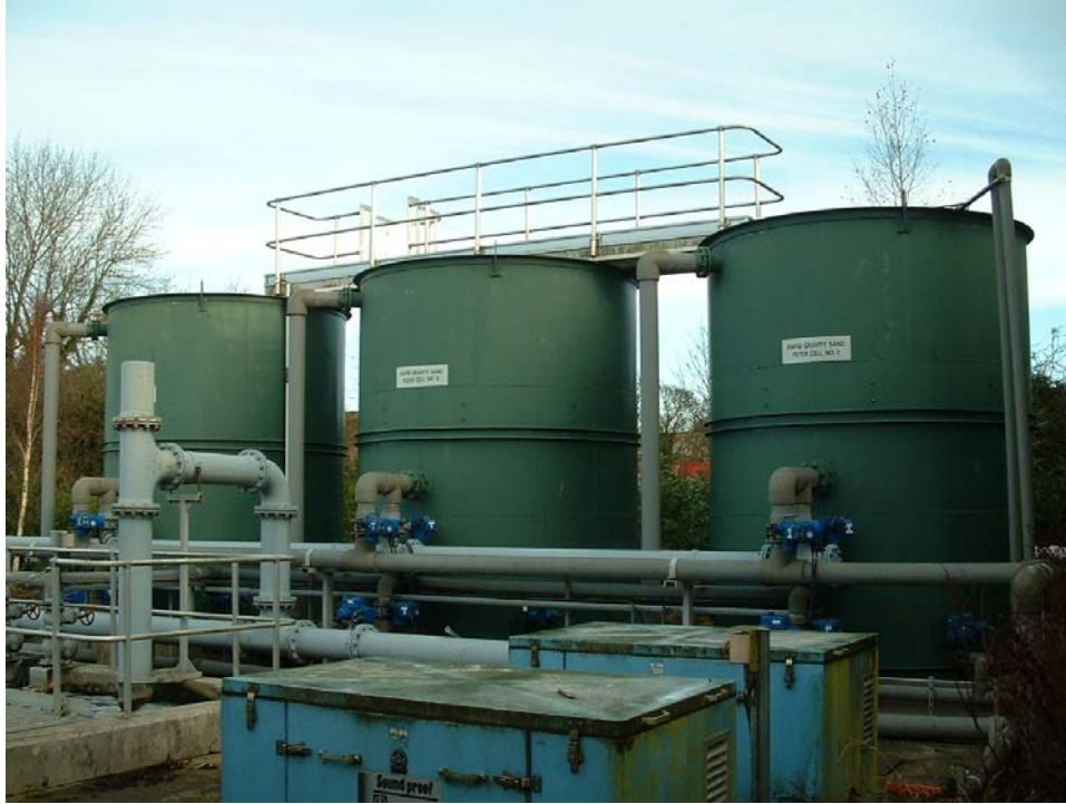
Photograph 1.2 – Existing effluent polishing filters at Carrickmacross
