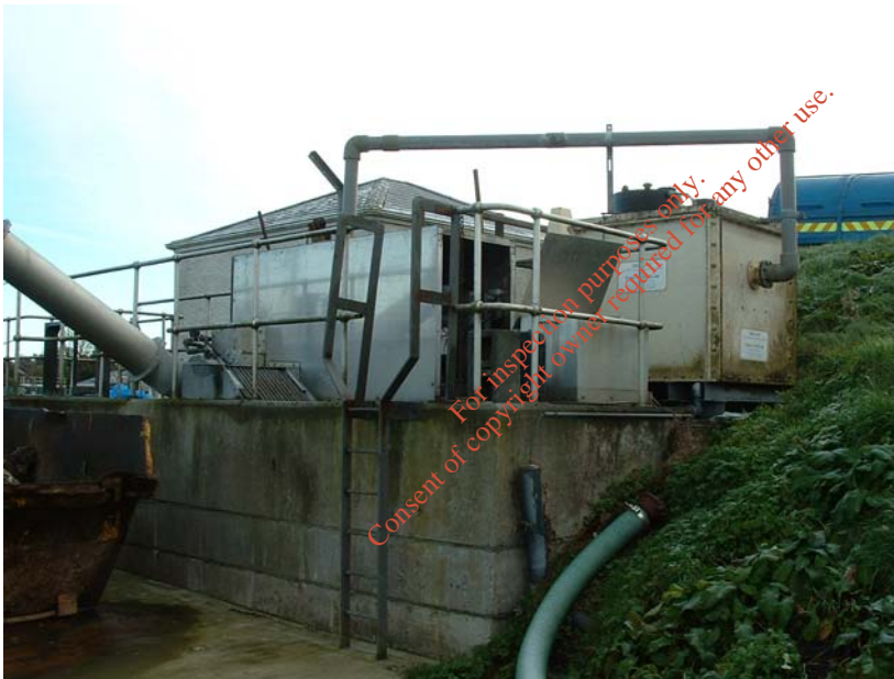
Photograph 3.11 – Inlet works with Odour Treatment
