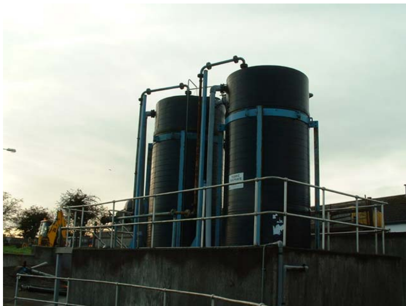
Photograph 3.5 – Ferric Sulphate Storage Tanks
