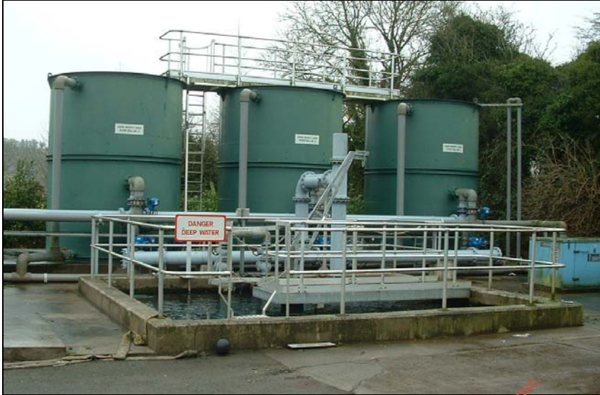
Photograph 3.7 - Tertiary Sand Filters
