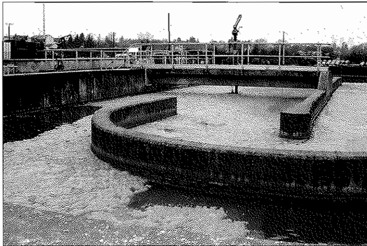
Fig. 2.04 – Oxidation Ditch No. 2
