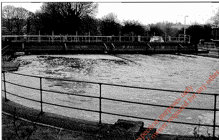
Fig. 2.03 – Oxidation Ditch No. 1
