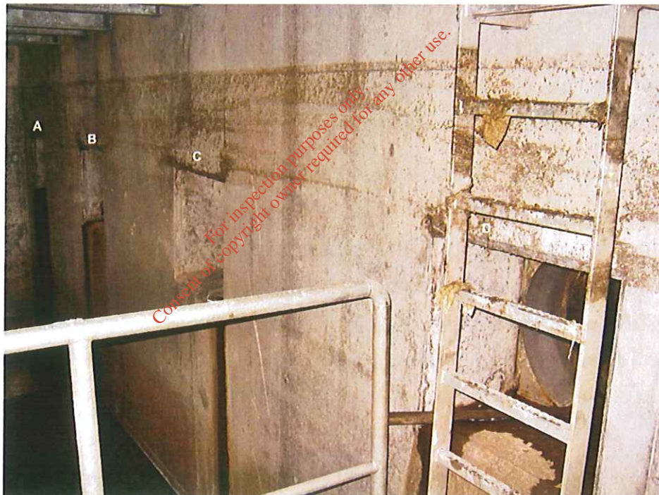
Fig. 4.16 Photo 1 – Pumping chamber showing the four gravity openings - A,B,C & D
