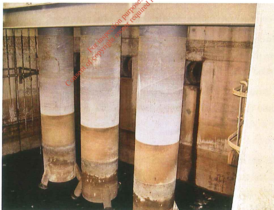
Fig. 4.18 Photo 3 – Pumping Chamber
