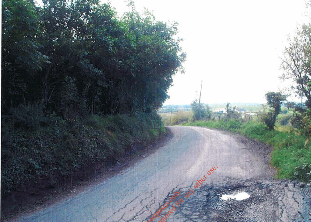
Plate 18.2 Road Surface Before Upgrading
