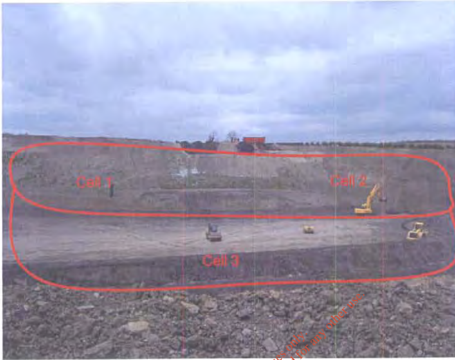
Plate 3.4.5: Engineered Cells May 2006
