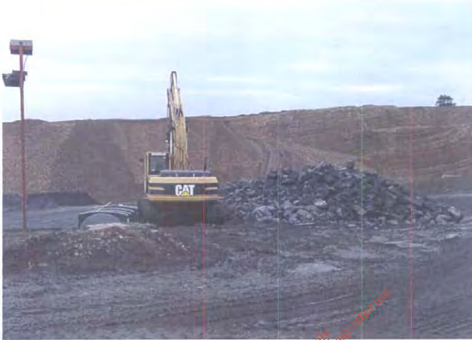
Plate 3.5.13: Crushing and Screening Plant from Internal Roads
