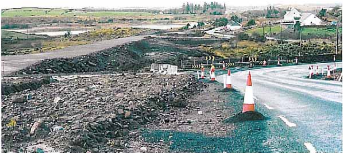
Plate 4. From Cartron to Cuilmore a section of new road of c.1 km is under construction. View is looking westwards.
