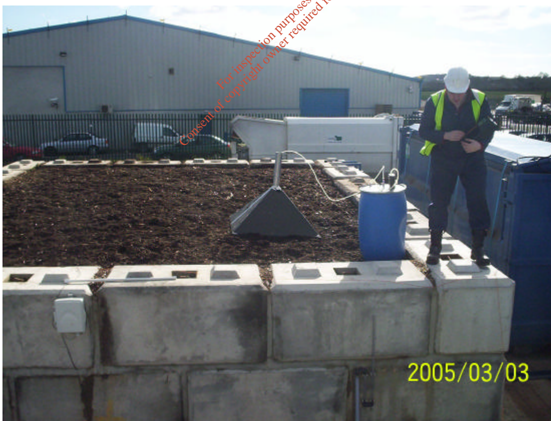
Figure 9.2. Overview of biofilter hood for capturing odours from the surface of the biofiltration systems. Additionally, the air distribution within the biofilter media was audited to check air distribution performance.
