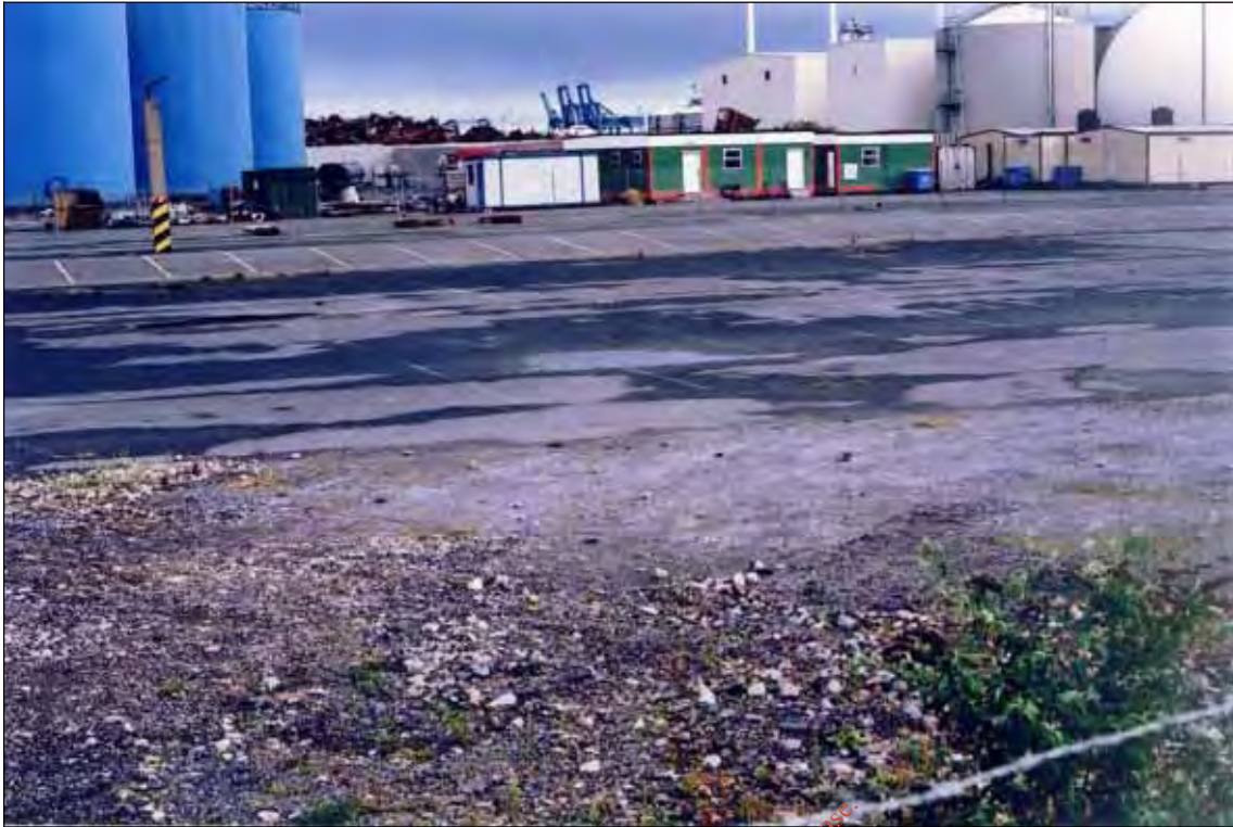
Plate 1: Cracks providing a niche for plant species
