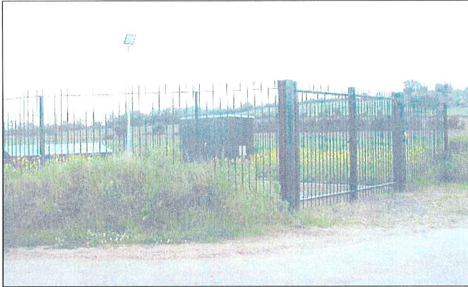
Figure 1: Production well 2 (PW2), showing the concrete platform, railings, well-head protection cabin and pump-control housing.
