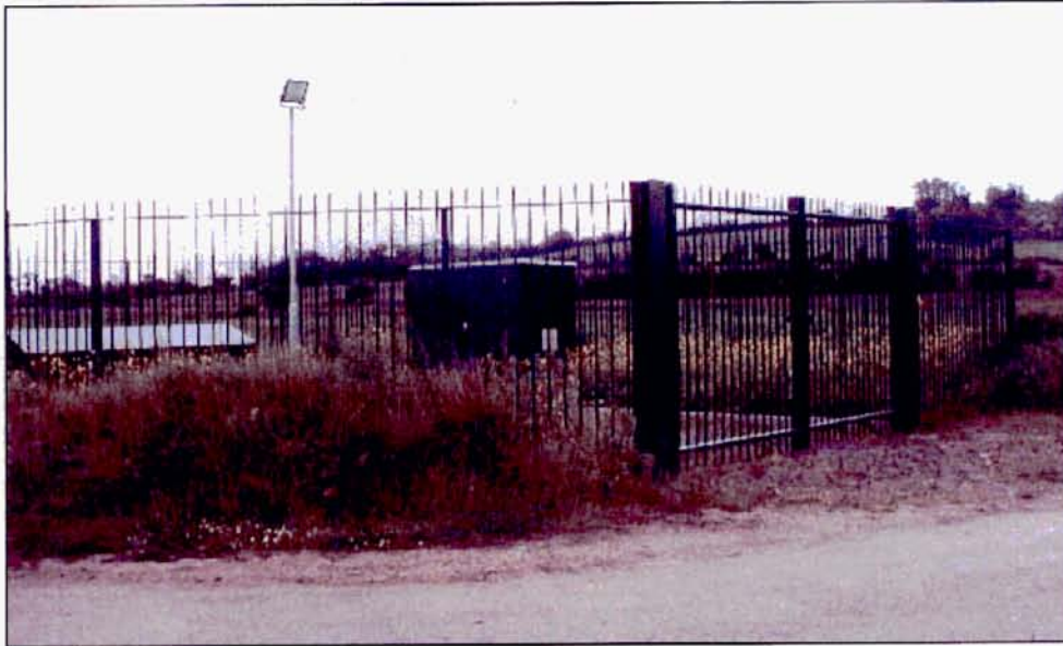
Figure 1: Production well 2 (PW2), showing the concrete platform, railings, well-head protection cabin and pump-control housing.
