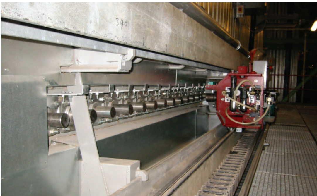
Figure A5.5 Mechanical rapping device at Elsam's Odense Waste to Energy Facility
