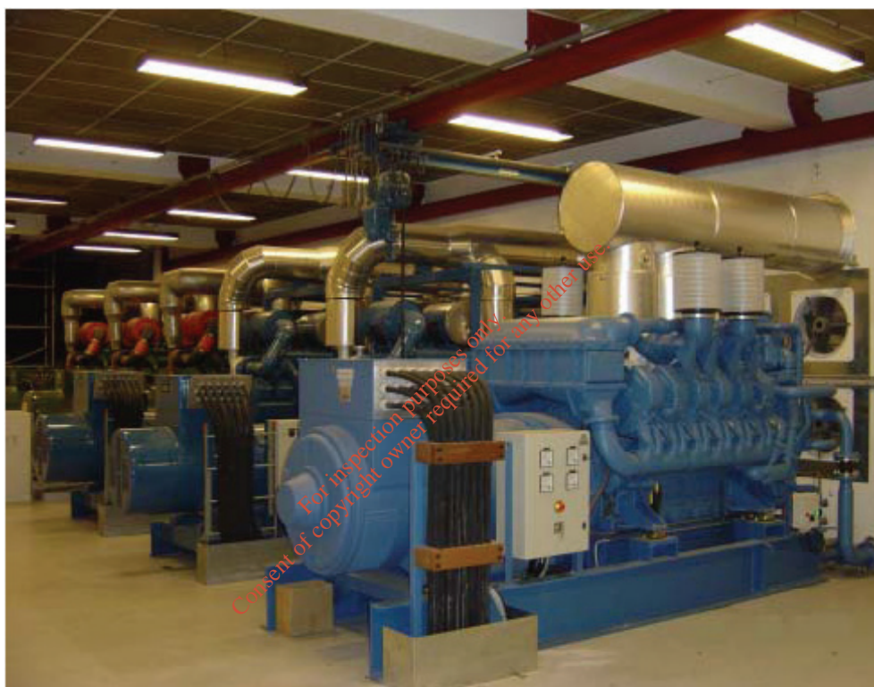
Figure 5.10 Emergency Diesel Generator
