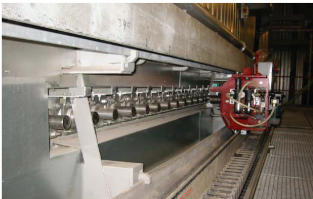
Figure 5.6 Rapping devices for cleaning of the horizontal pass at Elsam Odense WtE
