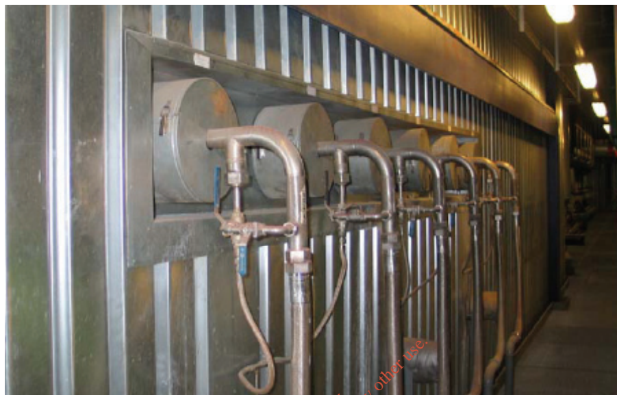
Figure 5.9 One SNCR injection level at Elsam Odense WtE Facility
