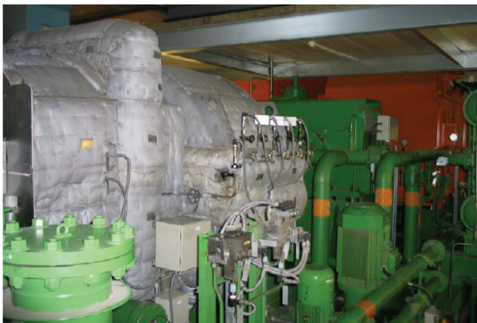
Figure 5.8 Turbine and generator set at Elsam Odense WtE
