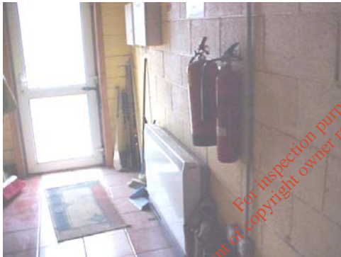
Plate J.1: Fire Extinguishers located by the entrance/exit of the Site Office
