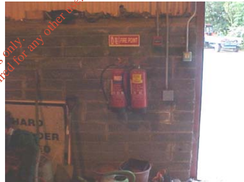
Plate J.2: Fire Extinguishers located in the garage building
