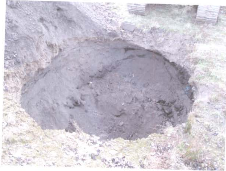
Photoview 2. Trial Pit 62 containing fines/soils
