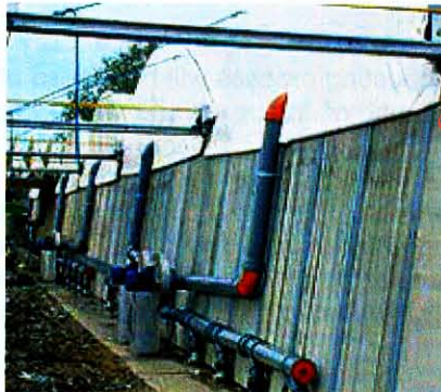
Plate 6 External air ducting and Fans
