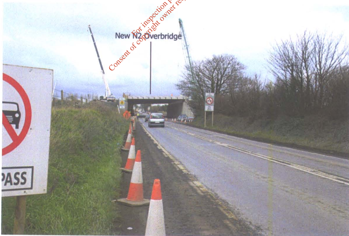
Photograph 14. View from N2 at proposed site entrance, looking to the north to the new N2 overbridge (under construction). The existing earth embankments will provide some screening of the site to road users.
