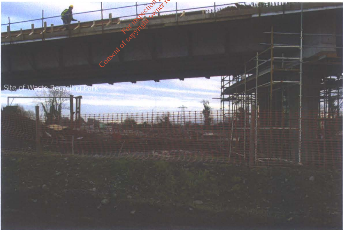
Photograph 6. View looking south from centerline of new N2 at site Kilshane road overbridge (under construction). The site is located in the middle left of this view. Intervening vegetation and approach earthworks of the new overbridge will screen the majority of the Waste Recycling Park from here.
