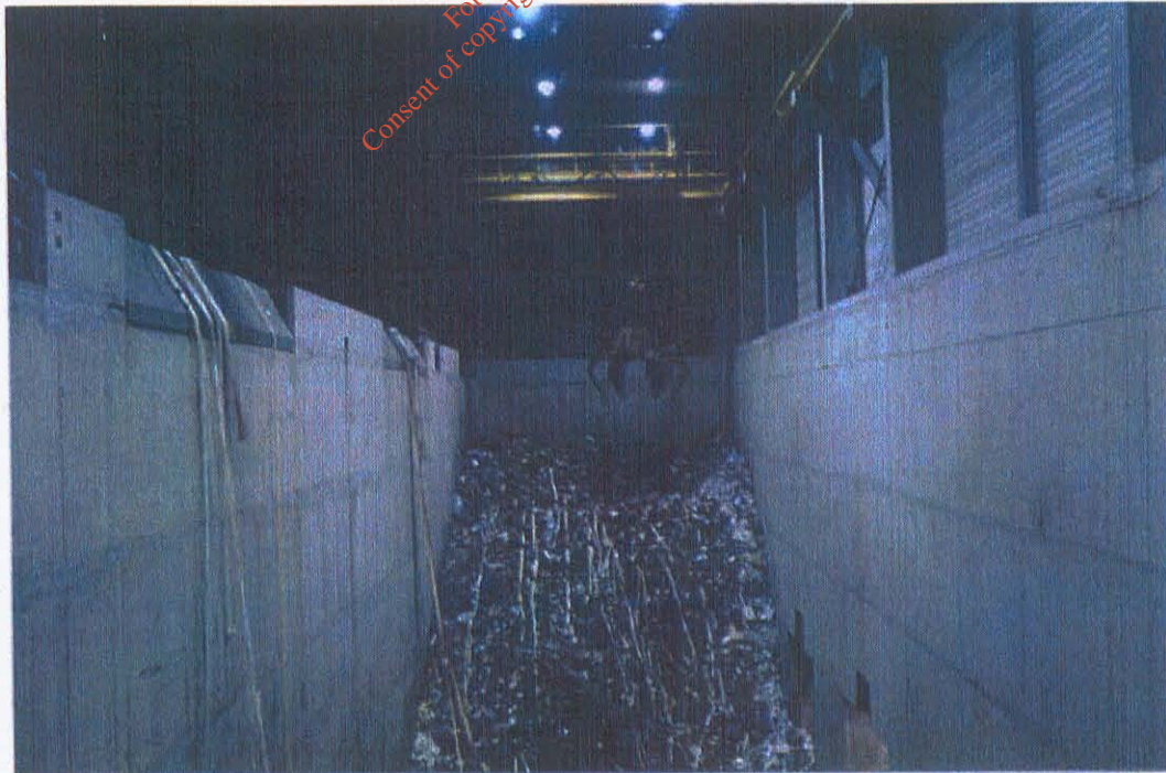
Grab Crane over Waste Bunker
