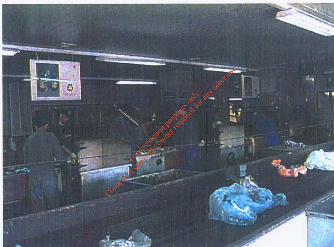
Typical Picking Station at Materials Recycling Facility
