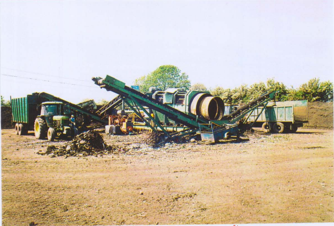
Photograph 11. View of the screening unit
