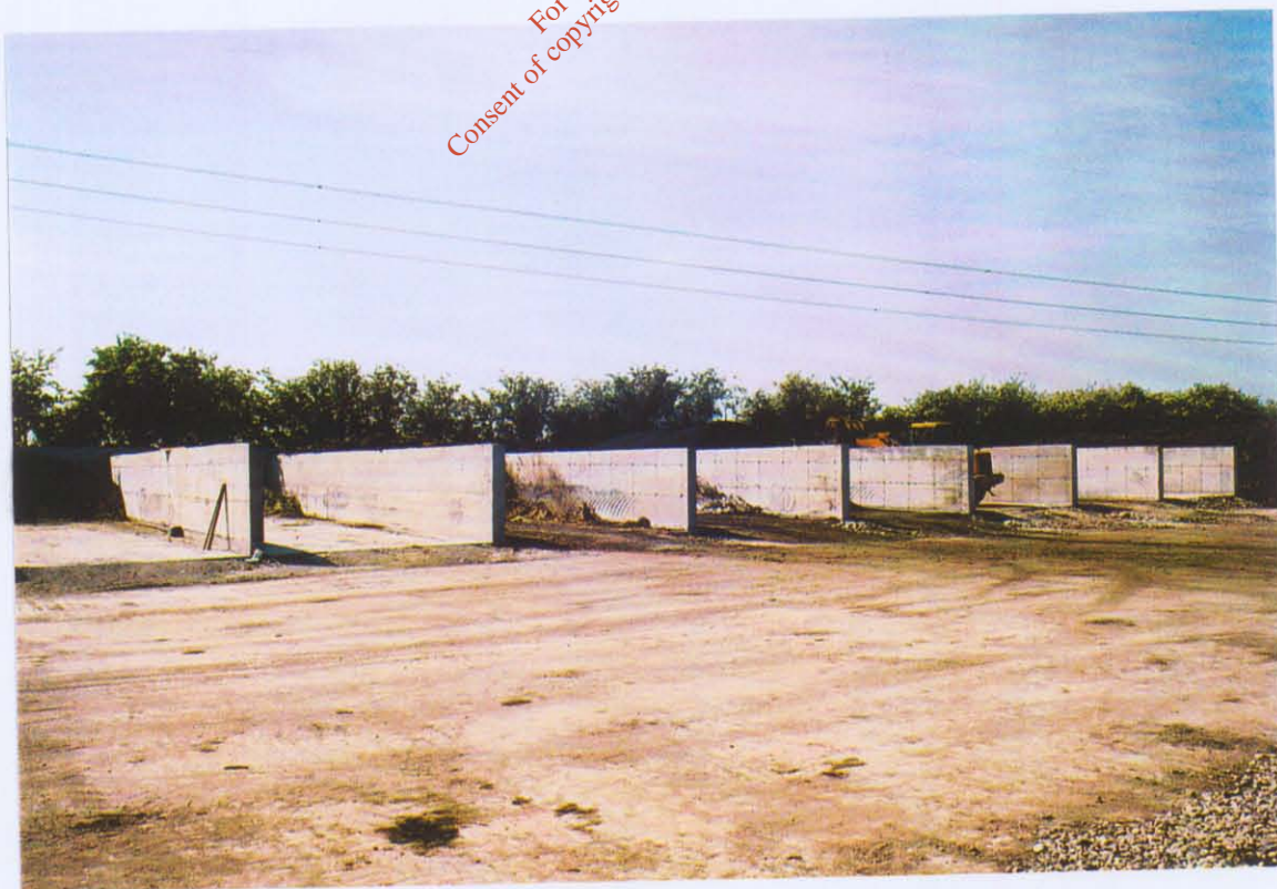
Photograph 10. View of the waste reception bays and the concrete base in front of them
